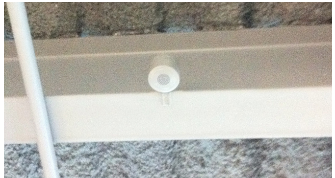
Qt emitter mounted onto an exposed steel beam in the open office area
